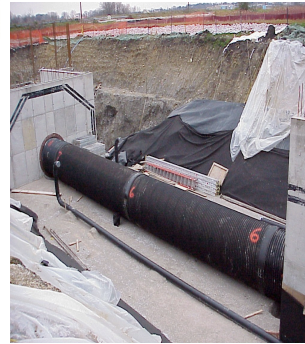
50-m decay pipe
